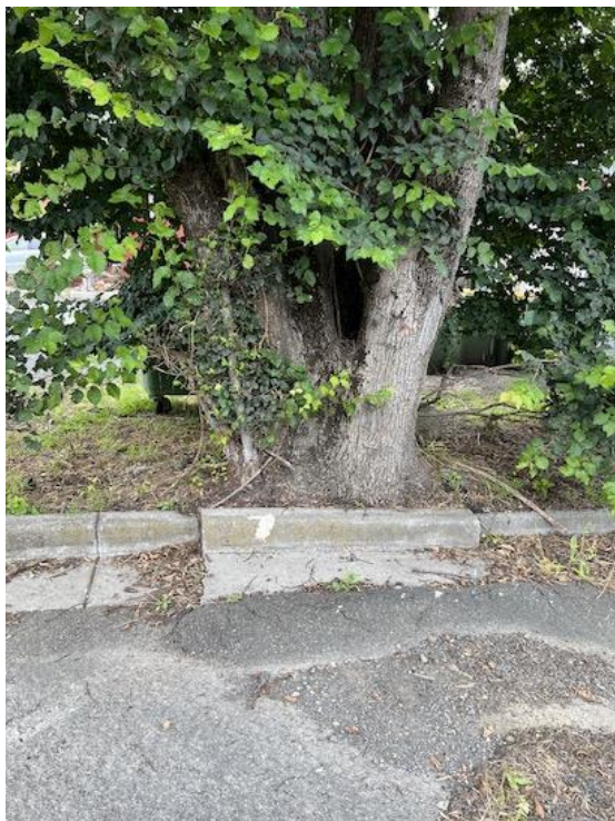
Tree 2 trunk roots cracking curbing & bitumen
